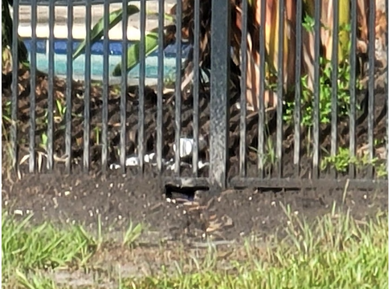
Photo 2 showing pvc pipe discharging to the CDD pond bank causing erosion.
